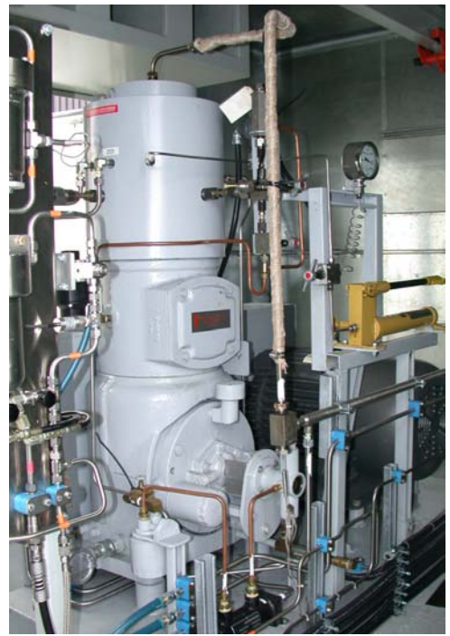
Figure 3: 25 scfm diaphragm 87.5 MPa compressor
