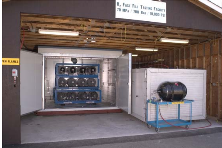
Figure 7: 70 MPa fast fill facility
